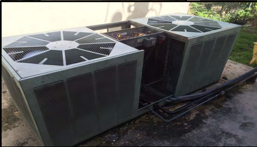
A/C unit at Fire Station 2
