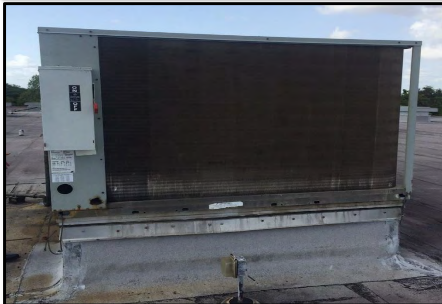
A/C unit at the 72nd Avenue complex
