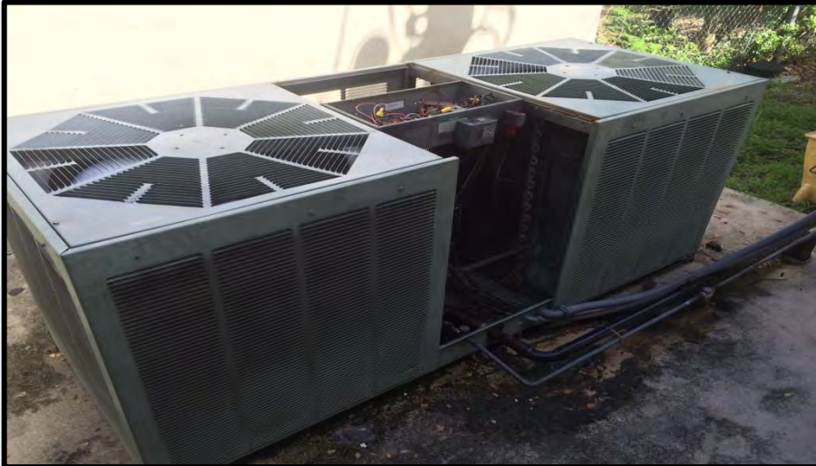
A/C unit at Fire Station 2
