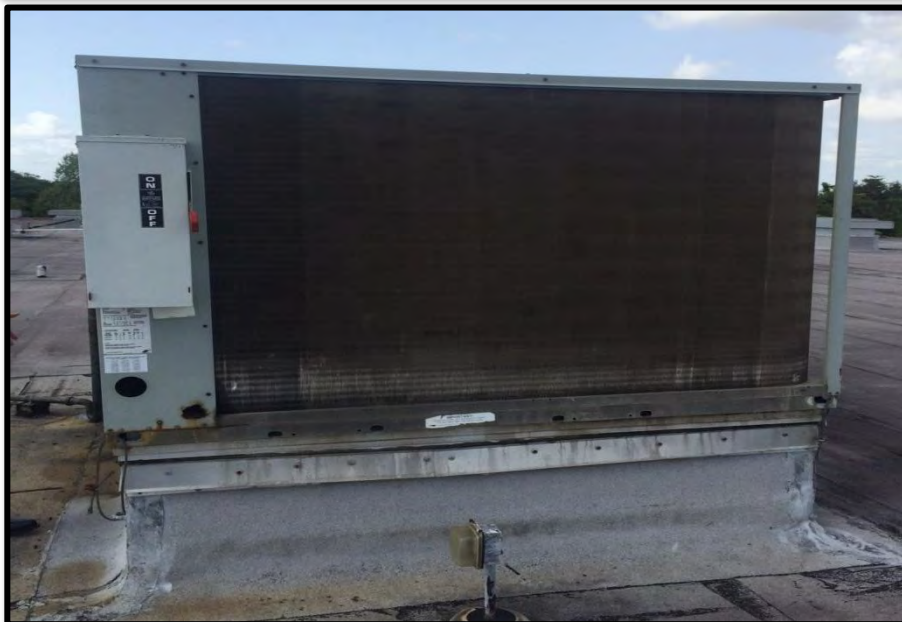
A/C unit at the 72nd Avenue complex
