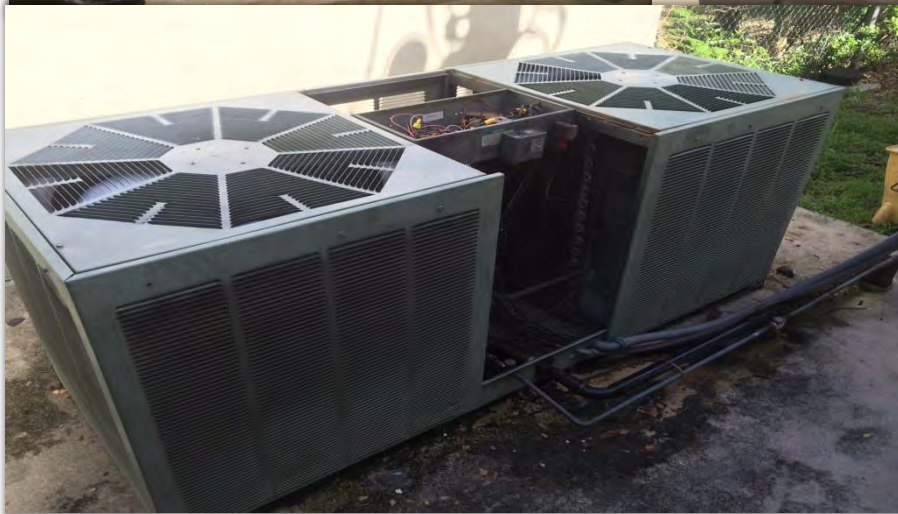
A/C unit at Fire Station 2
