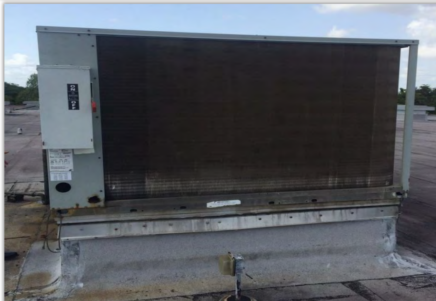
A/C unit at the 72nd Avenue complex
