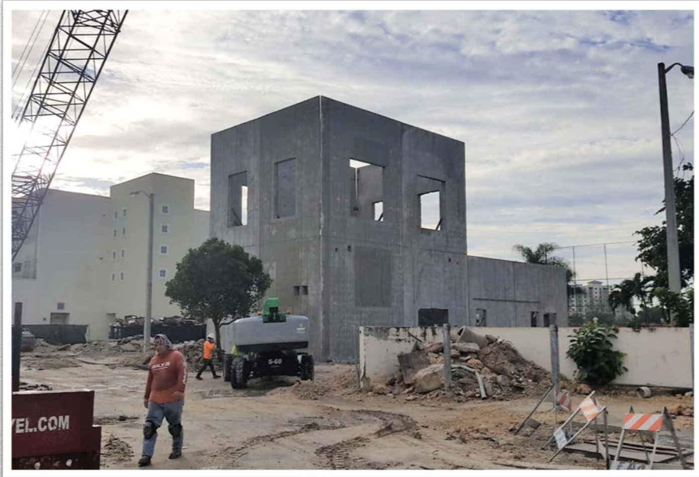
New Central Chiller Plant – (Riviera Drive)
